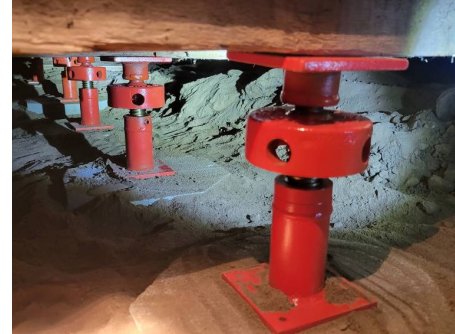
Footings & jack posts were installed and soil contact with joists mitigated in the crawl space
